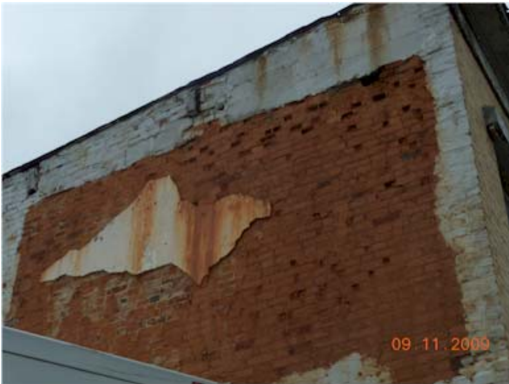
Figure 4 Exposed party wall and deteriorating bricks
